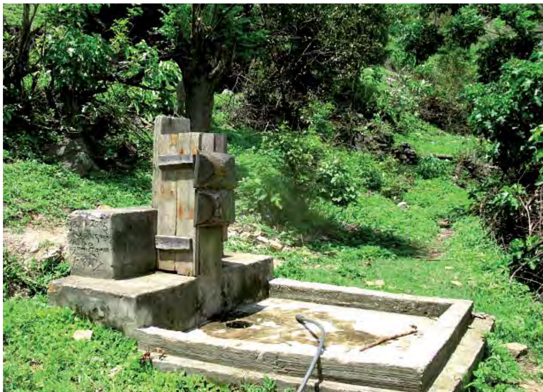
Not a done deal: Renovation works are left incomplete in Dremetse
